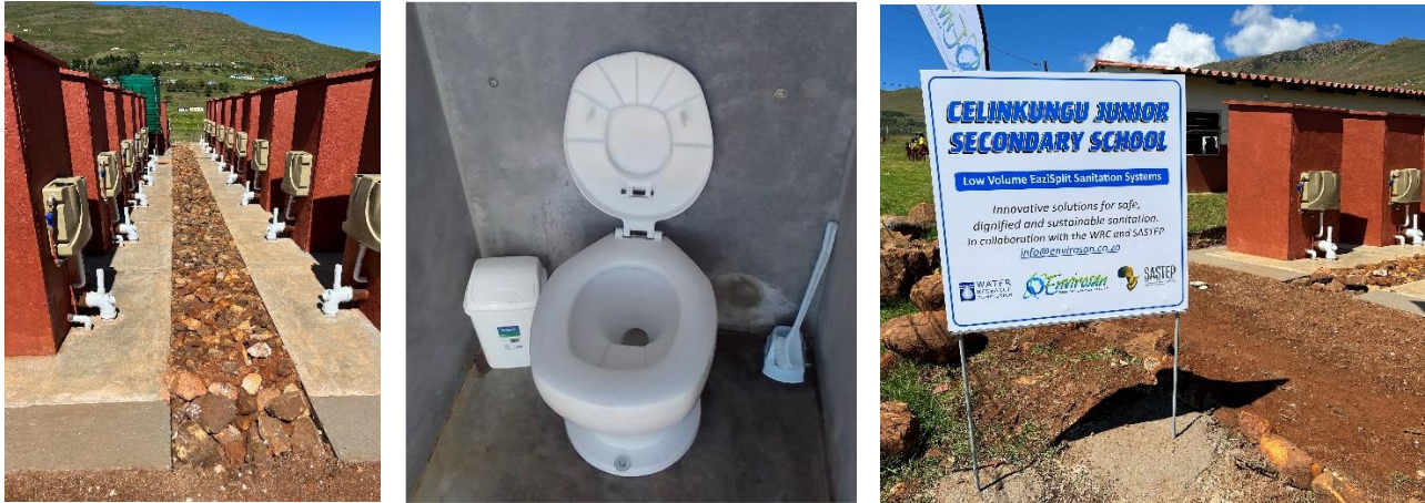
Figures 1-3: EaziSplit™ Sanitation System installed at Celinkungu Junior Secondary School
